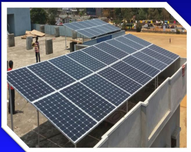
10 kW Off-Grid Solar Power Plant Venue: Bhandarkars' Arts and Science College, Kundapura, Karnataka
