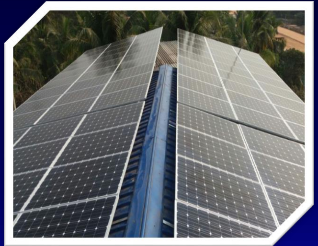
40 kW Off-Grid Solar Power Plant Venue: Dr. NR Acharya Memorial Hospital, Koteshwara, Karnataka
